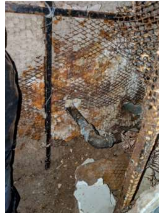
Missing insulation on cold water supply t
